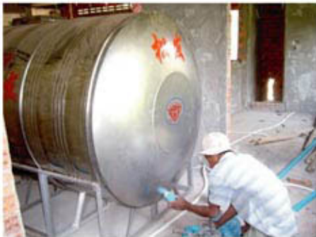
Water tank being installed inside the orphanage. Clean fresh water insures that the children will not be exposed to water born illness.
