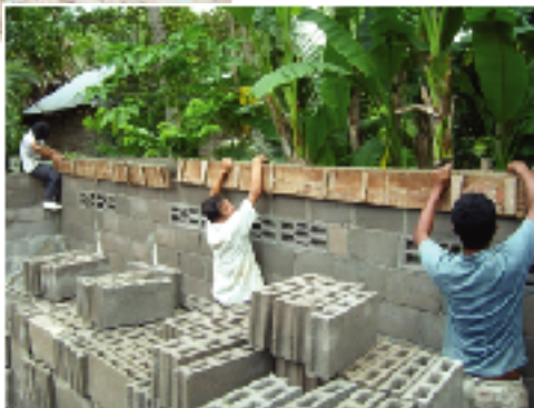
The perimeter wall is constructed and forms are put in place to pour a concrete header.
